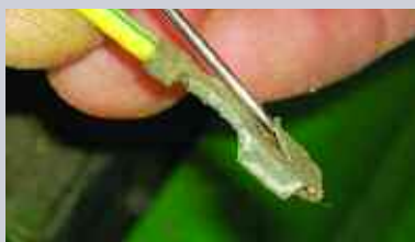
Inspect plugs and sockets regularly for damage, loose wires and bent pins.
