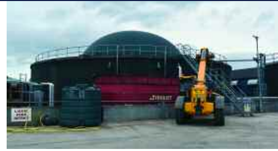
Following the installation of the AD plant, the farm quickly realised they were generating a lot of additional heat from the engines which could be used to their advantage.
