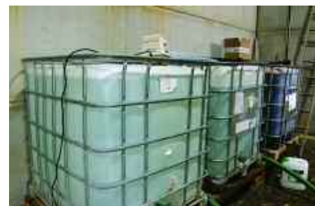
The series of IBCs are used to brew microbes from a concentrate that are then added to the spray tank.
