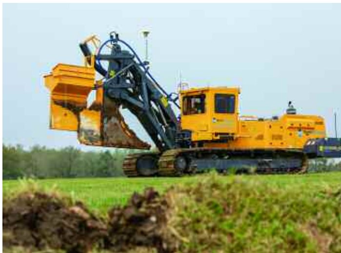
Rob Burtonshaw will discuss how cleaning ditches and clearing outfalls is a simple and cheap way of improving the efficiency of the drainage system.
