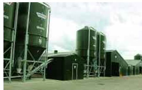
At the heart of the business lies a state-of-the-art 190,000-broiler unit, serviced with ground-source heat pumps and solar panels.
