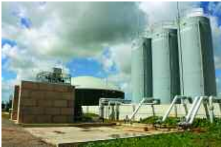
Three tall siloes store a share of the 25,000t/yr of food waste that makes up around 50% of the digester’s diet.
